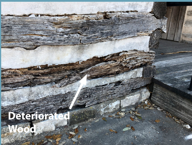
FIG. 5: Loss of wood due to fungus.
