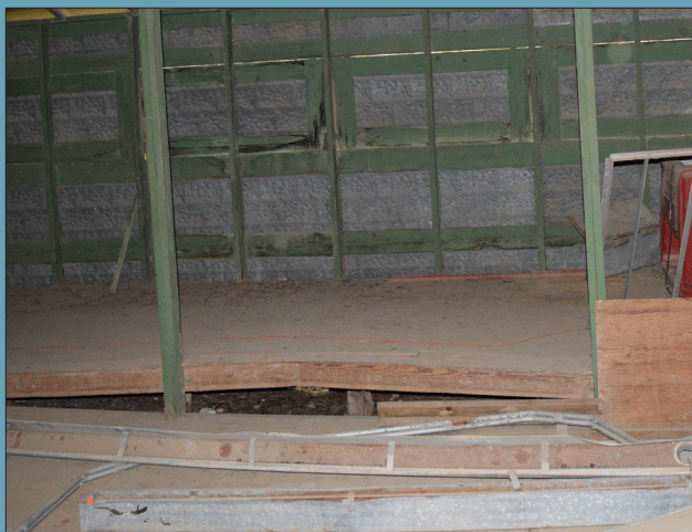
FIG. 54: Floor to left of the center post is buckling upward, which may be result of leaking roof or shift in the foundation.
