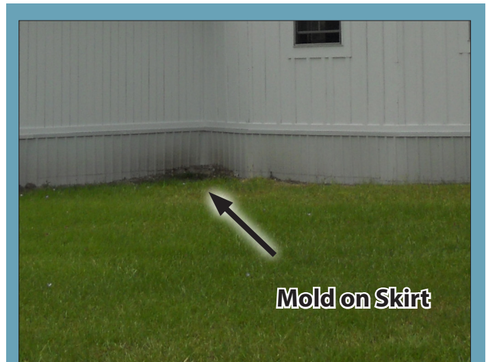
FIG. 27: Mold on skirting indicates excessive moisture and ventilation issues maybe present under the dance hall.
