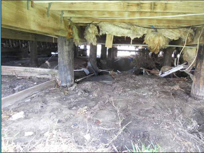
FIG. 29: Water erosion due to flooding under dance hall.
