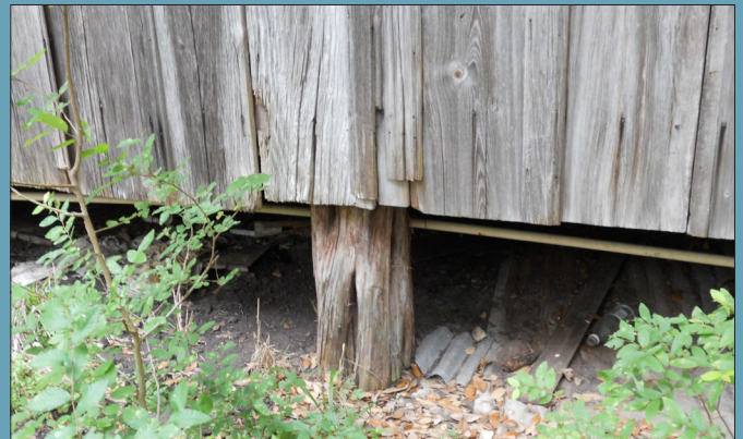
FIG. 22: Wood foundation post on ground exposed to active water. Keep dry to prevent rot. Note rotting post.
