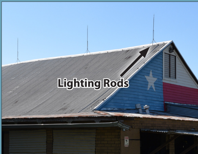
FIG. 65: Lightning rods on roof.
