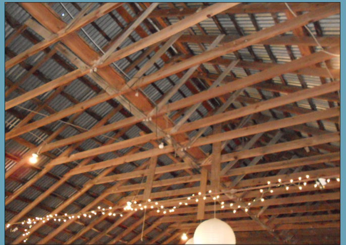
FIG. 41: Rafters or joists are spaced further apart than modern construction. Look for sagging beams or ridge lines.
