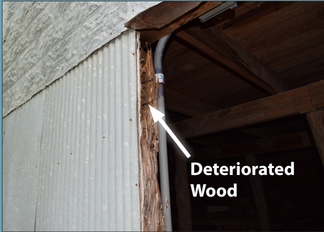
FIG. 3: Deteriorated structure from dry rot.
