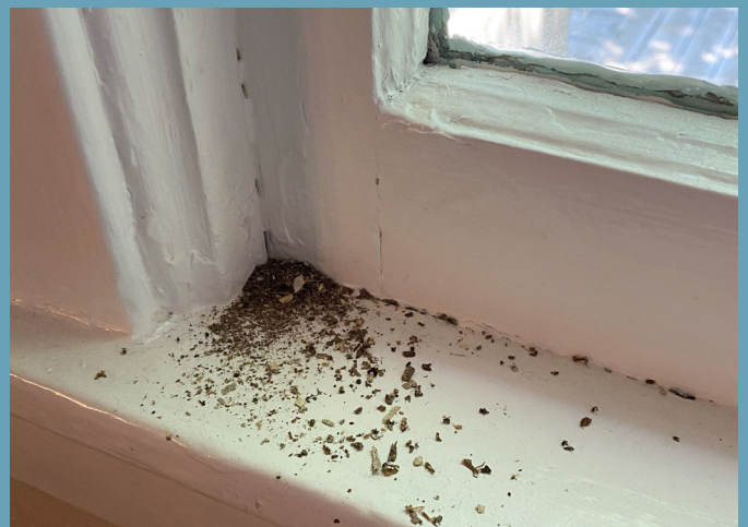
FIG. 8: Carpenter ant frass appears as saw dust.
