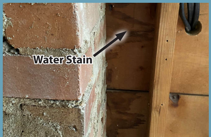
FIG. 37: Water stain indicates leak. Repair leak and allow wood to dry. No wood stabilization is needed as the element is intact.
