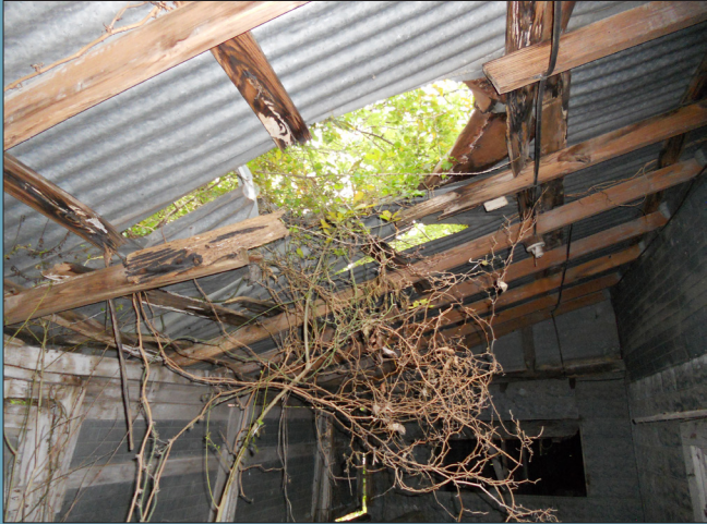
FIG. 49: Holes in the roof need immediate repair.
