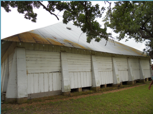
FIG. 17: Rust present under drip line of tree.
