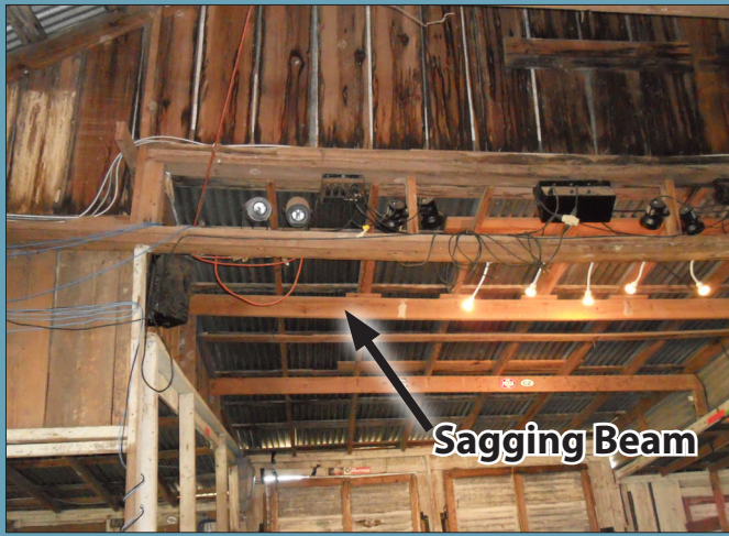
FIG. 33: Bearing wall removed to expand stage. Note sagging beam, add support post.
