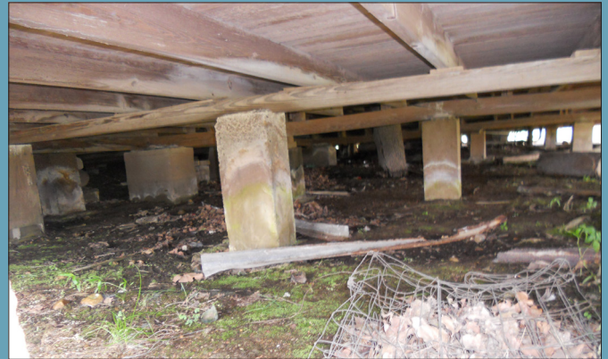
FIG. 21: Shifting foundation may place support columns at awkward angles. Monitor with plumb bob from top of post.
