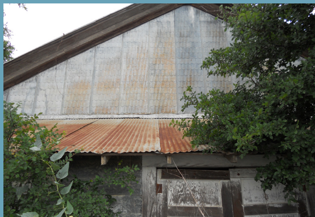
FIG. 18: Rusting but stable sheet metal.
