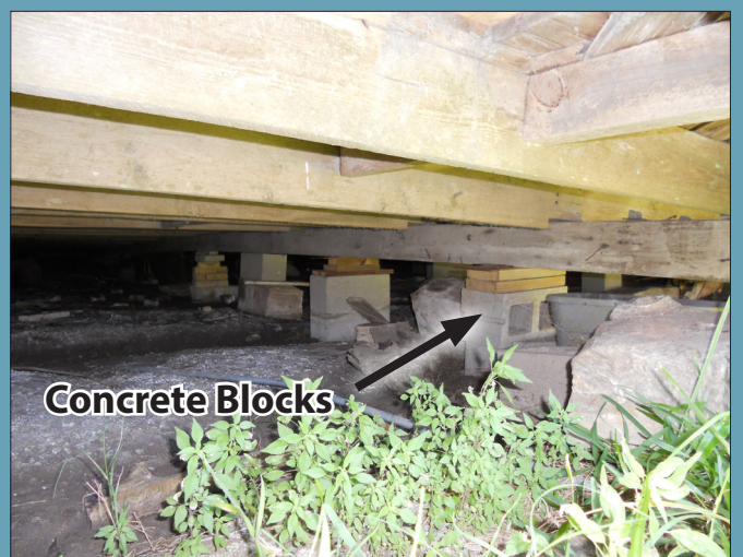
FIG. 23: Inadequate footing: concrete blocks can collapse.
