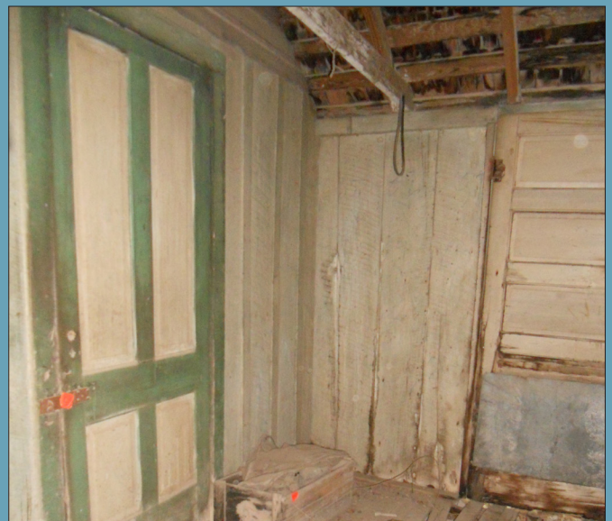
FIG. 35: Deteriorating bearing walls. Note damage to the floor as well.
