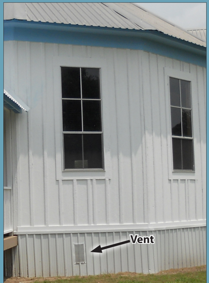
FIG. 28: A larger vent is recommended to increase air circulation within the foundation and under the dance hall.
