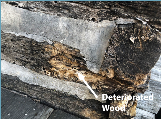
FIG. 4: Loss of wood due to fungus.
