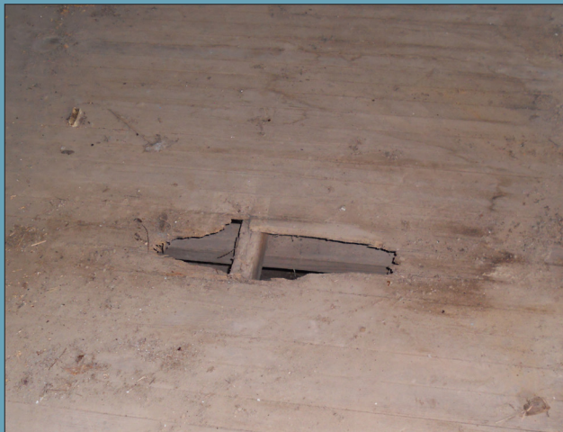
FIG. 53: Hole in the floor caused by leaking roof.
