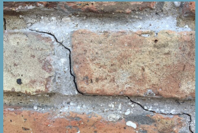
FIG. 15: Hairline cracks through mortar joints indicate slight movement and should be monitored.
