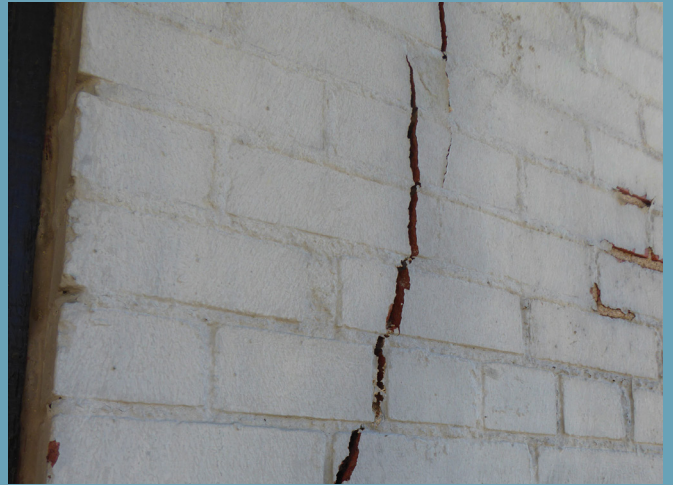
FIG. 14: Cracks through brick units indicate structural movement and instability.
