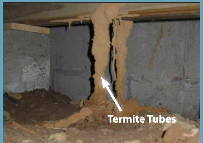
FIG. 7: Termite tubes leading to underside of structure.
