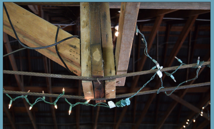
FIG. 42: In this case, a column was removed and the structure now bears on steel cable. This modification may compromise the structure and should be evaluated by a professional.
