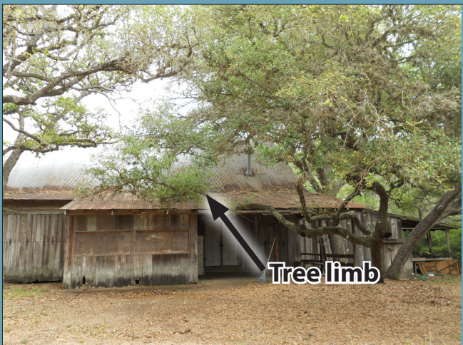
FIG. 61: Trees leaning on roof.
