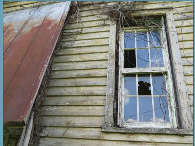
FIG. 62: Broken windows on abandoned building.
