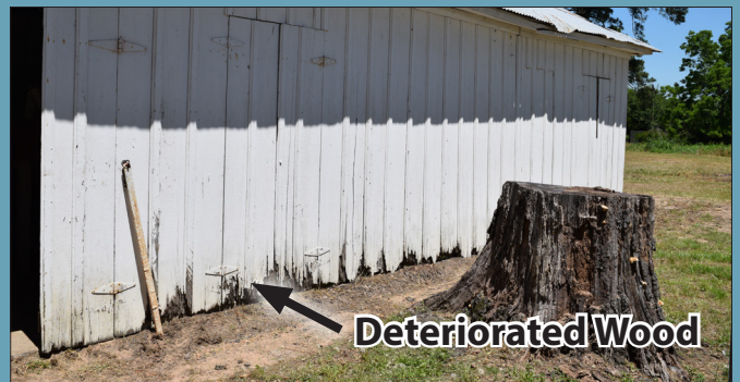
FIG. 36: Deteriorated wood siding allowing water into building.
