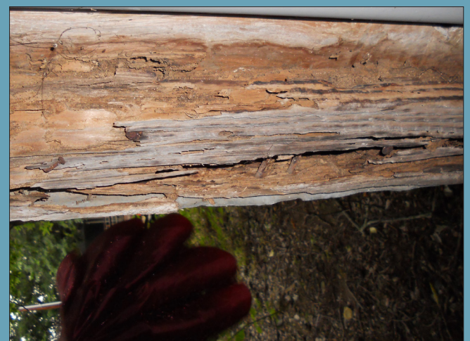
FIG. 48: Deterioration of wood member due to water damage or bugs.
