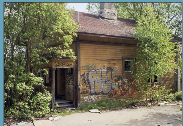
FIG. 64: Graffiti on abandoned building.
