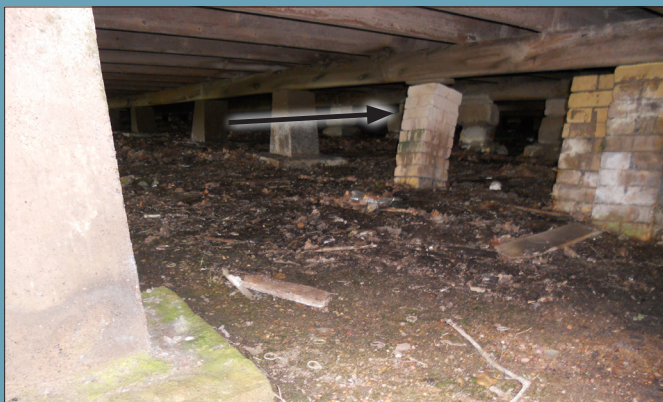
FIG. 24: Unsupported beam due to shifted column. Note brick post above has shifted, causing unsupported beam.
